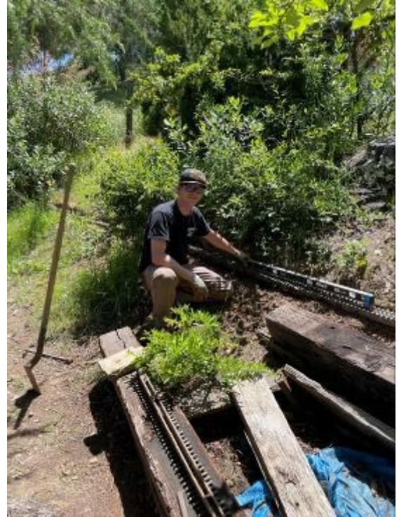
Jason Schoenmann checking the grade as he helps put 50 feet of track back in at a correct 1.5% climb.
