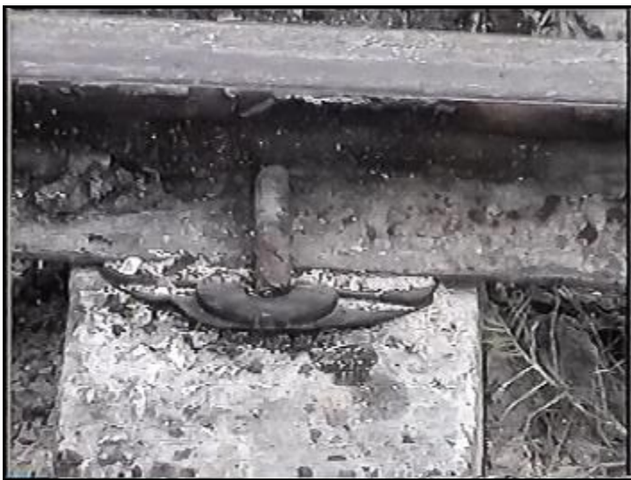
Wood for tie replacement is not available. New concrete ties have rebar anchors.
