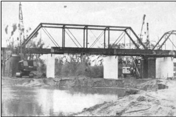
Project viewed from the east showing girder spans on temporary placements, awaiting movement of truss spans onto temporary wooden falsework.
