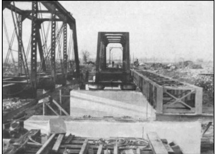
Northerly view from wooden trestle shows first truss span already moved onto falsework.
