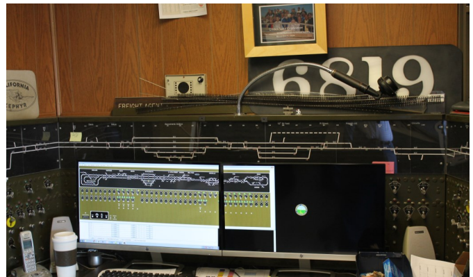
Dispatcher's Office and CTC Panel
