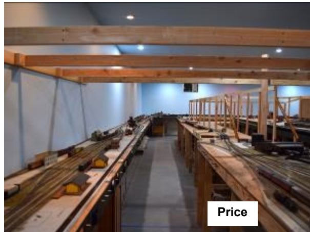
And The Rest Of The Addition Note The Upper Level Benchwork Under Construction (photo Ethan Doty)
